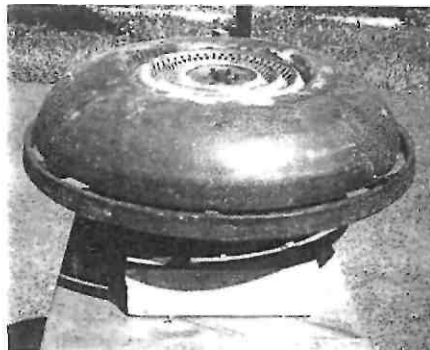
(c) Inner distributor cone removed to expose central portion of upper meander-plate.
